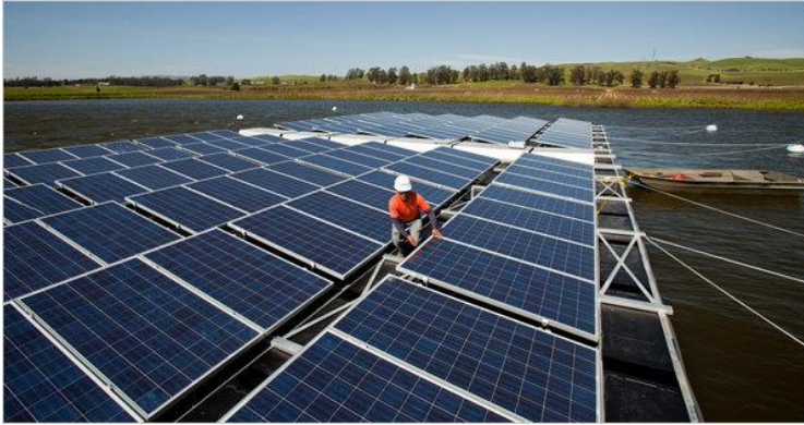
Figure 2. Sonoma County 200kW Floating Solar Array Example at Far Niente Winery
